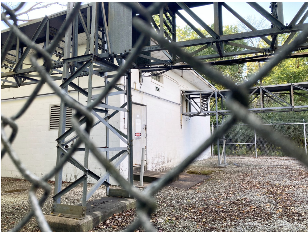
The original (1953) white block portion of the base station, which is the northwestern part of the structure.
