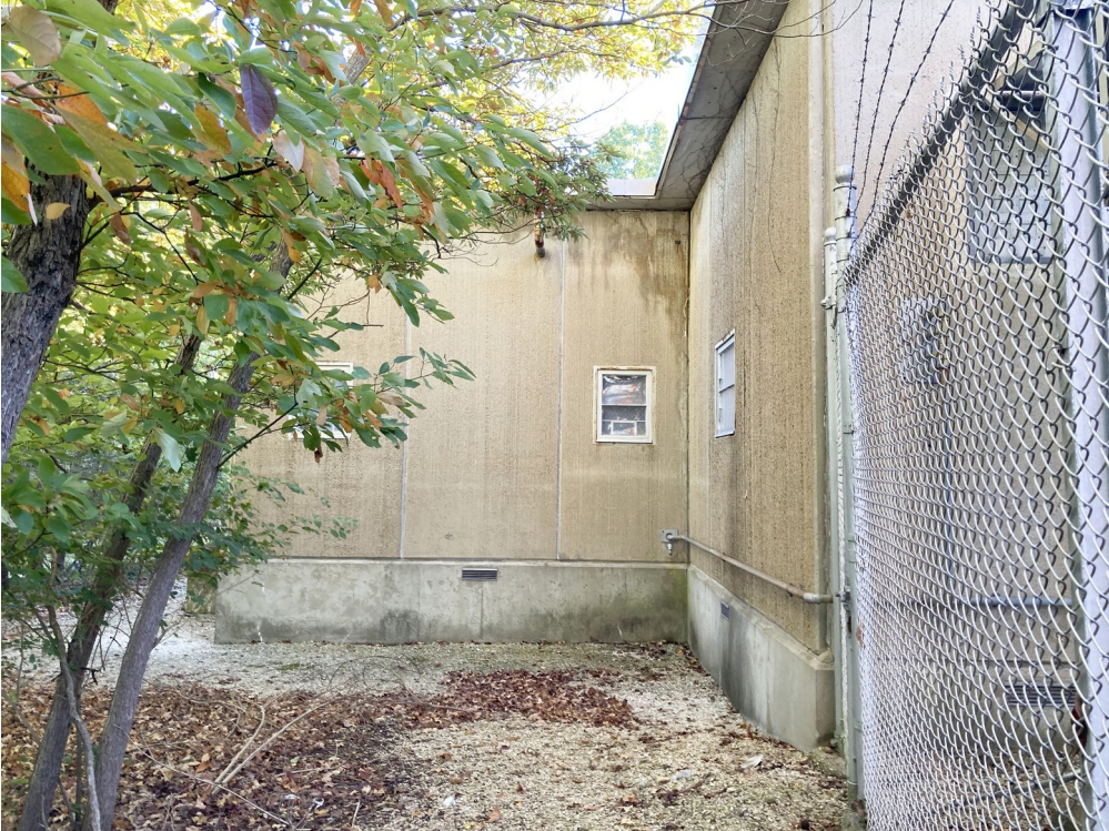
Part of the “semi-hardened” solid concrete addition, which was built around the southern edge of the original base station structure.
